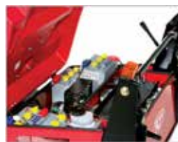
4 x 6v-180ah (5h) batteries
